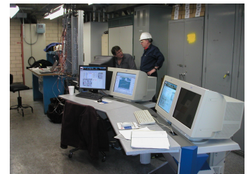
Avon Lake Unit 9 Operator Training Facility
